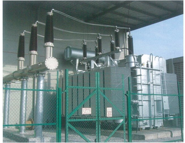
132/33kV 90/125MVA Power Transformer
