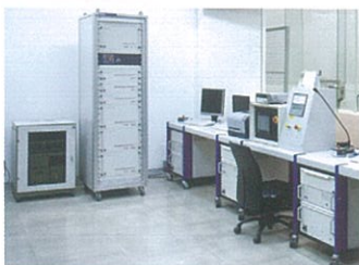
Control rack and Control desk TMS 580, 100kV 2000A
